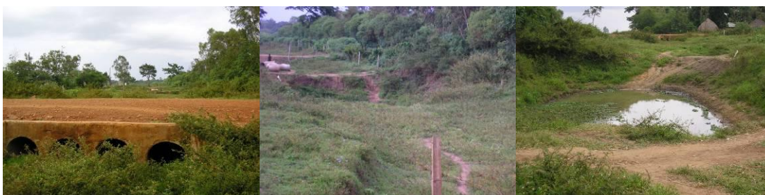
Pic. 17,18,19, shows different sections of the trench in Makunda. The first showing the drainage system to allow flood water not to disrupt transportation, the second showing the structure of the trench with water compartments and the third, a zoomed in water compartment which could potentially be used for irrigation
