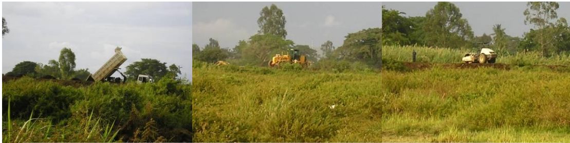
Pic. 13, 14, 15, showing the ongoing work of topping up the dyke at its weak point in Makunda. The first track brings in soil for topping, the second spreads it and the third compresses it.
